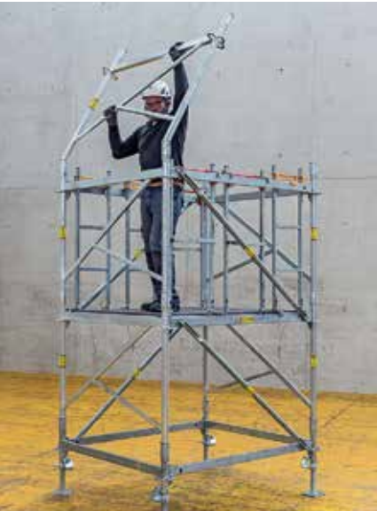
After attaching the frame to the tulip under 45°, the frame is turned into a vertical position.
